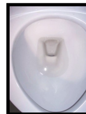
Clean Toilet Bowl After
