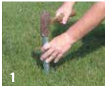
1 Drive the installation tool into the ground with a hammer at the starting point.
